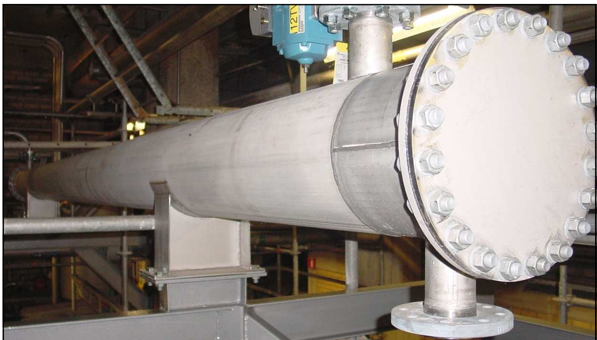
Twisted tube heat exchanger, AlfaTwist, in 1.4404/316L, during installation in a paper mill in central Sweden.
