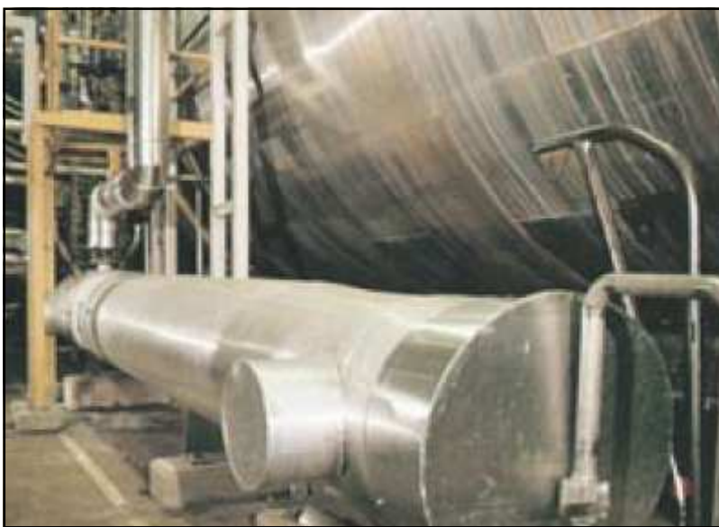
Thick liquor hea- ter in a paper mill in Sweden
