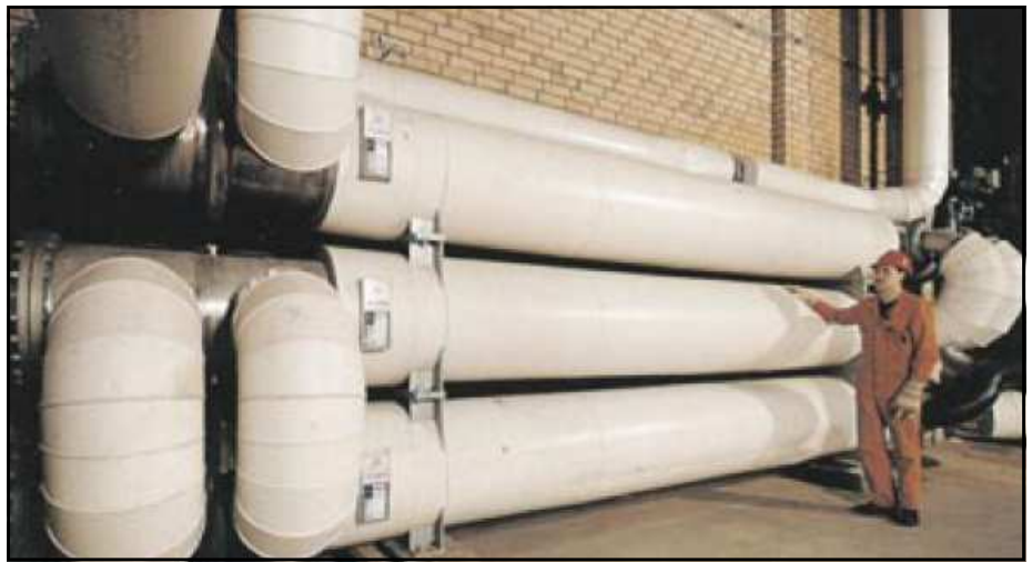
Liquor cooler in a paper mill in Sweden
